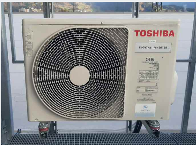
External air conditioning unit on wall bracket
